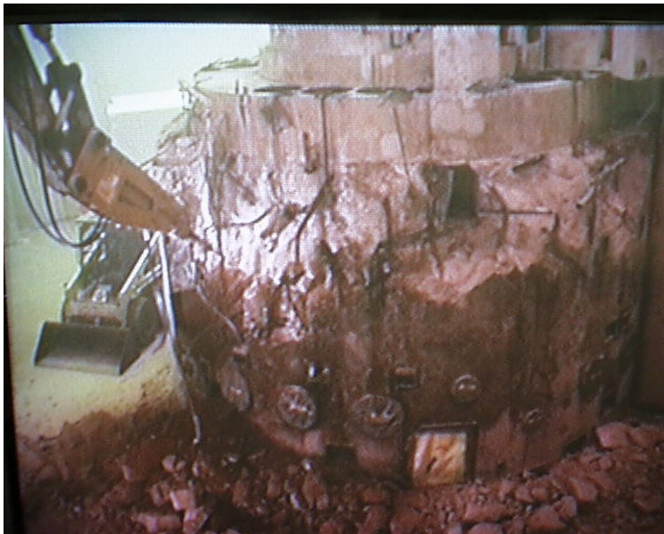
Figure 4. Georgia Tech used the 10 CFR 50.59 process to evaluate the safety impacts for dismantling the reactor bioshield instead of only removing the radioactive components. This action saved considerable time and money in the overall decommissioning process.
