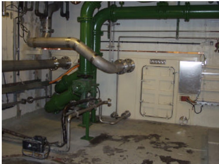
Photo. 2: Bulkheads with feeds through
