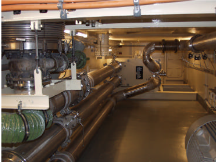
Photo 1: Coolant cycles with heat exchanger and bulkhead
