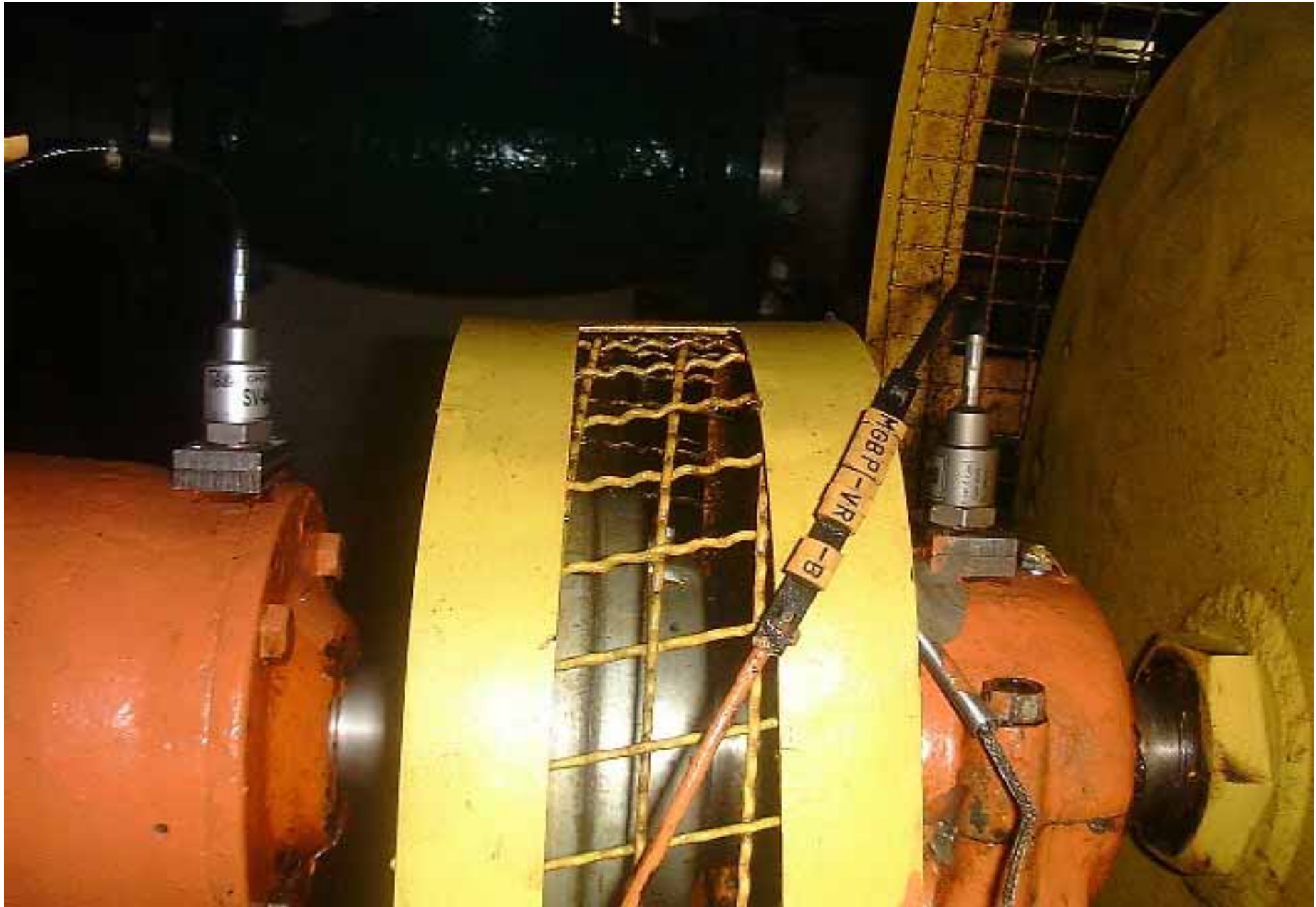
Bearings and accelerometers of the B Pump
