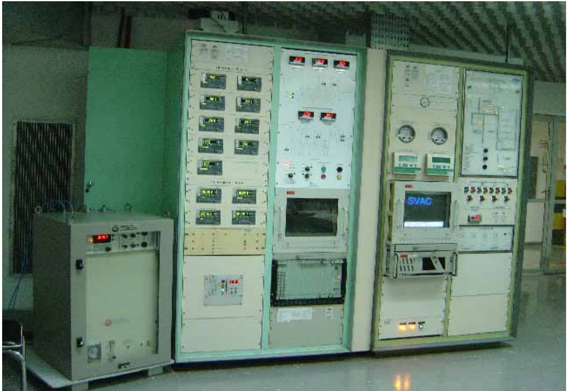
Some panels at the Control Room
