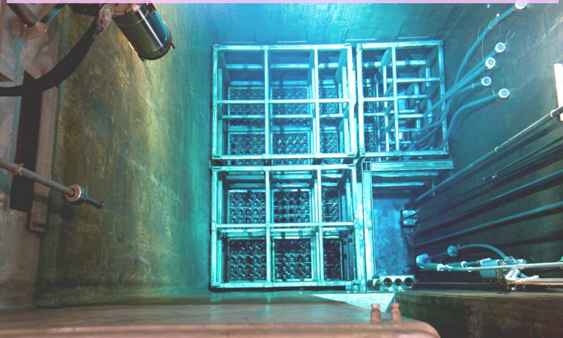
HANARO Spent Fuel Storage
