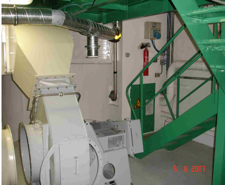
The new nuclear ventilation system
