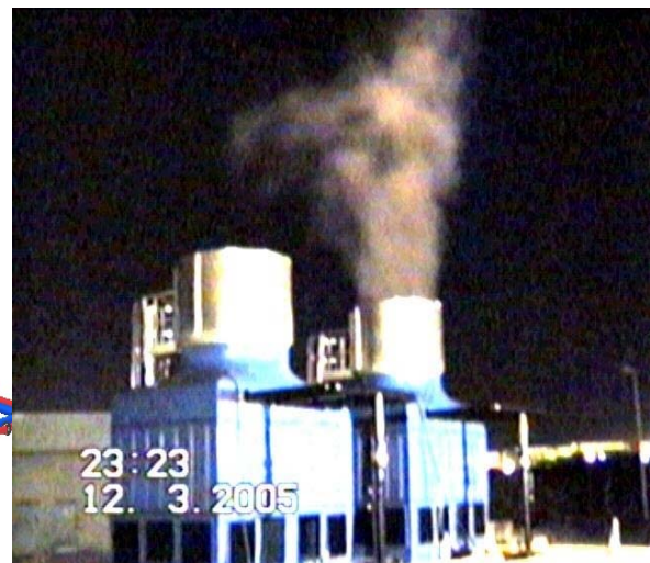
FIG.11. New cooling towers operating
