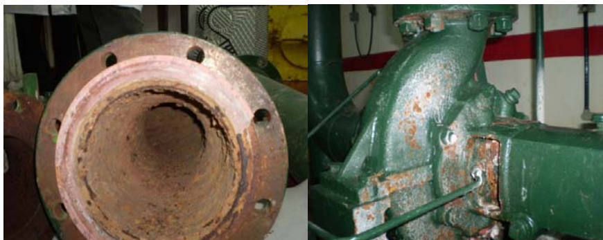
FIG.8. Corrosion/erosion of standard pipes of secondary loop
