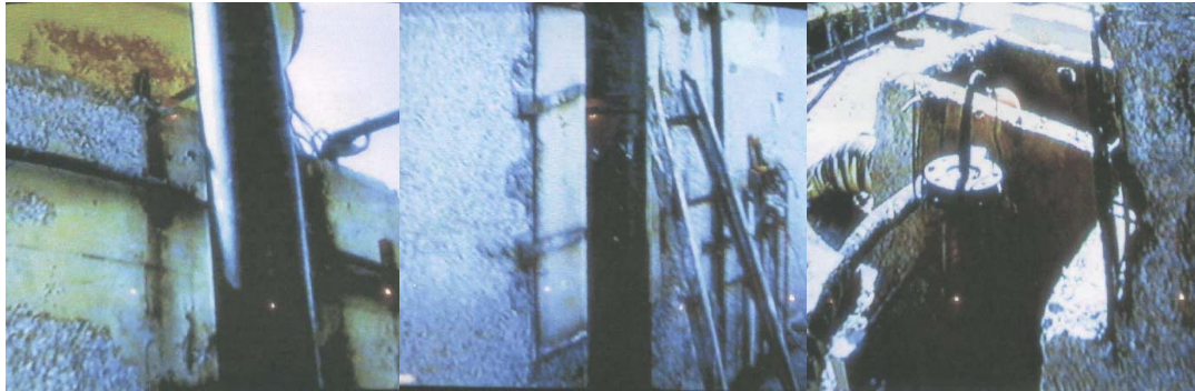
FIG.9. Cooling Tower degradation
