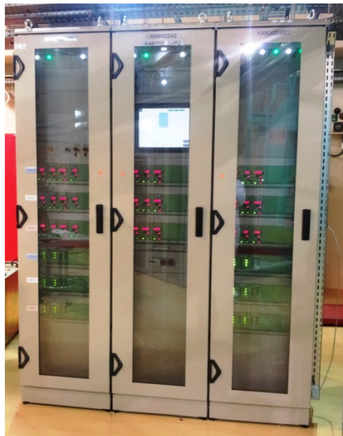
Figure 5 - CHOUCA SUR cabinet installed in OSIRIS reactor
