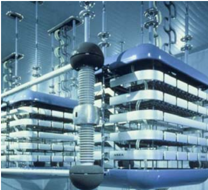
Fig 5: Example of high-voltage direct current (HVDC) system built from thyristors or hundreds of IGBTs
