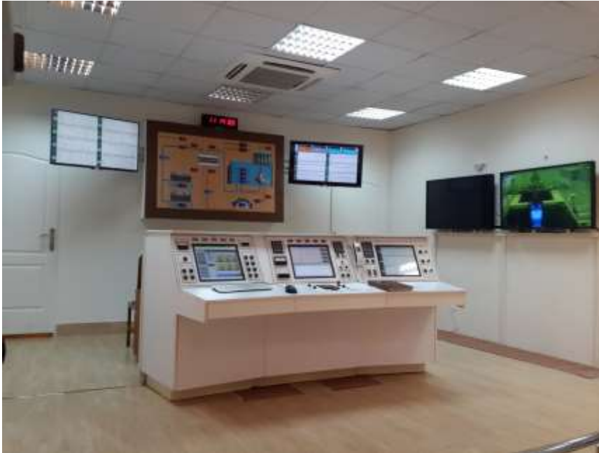
FIG.4. new control room of TRR
