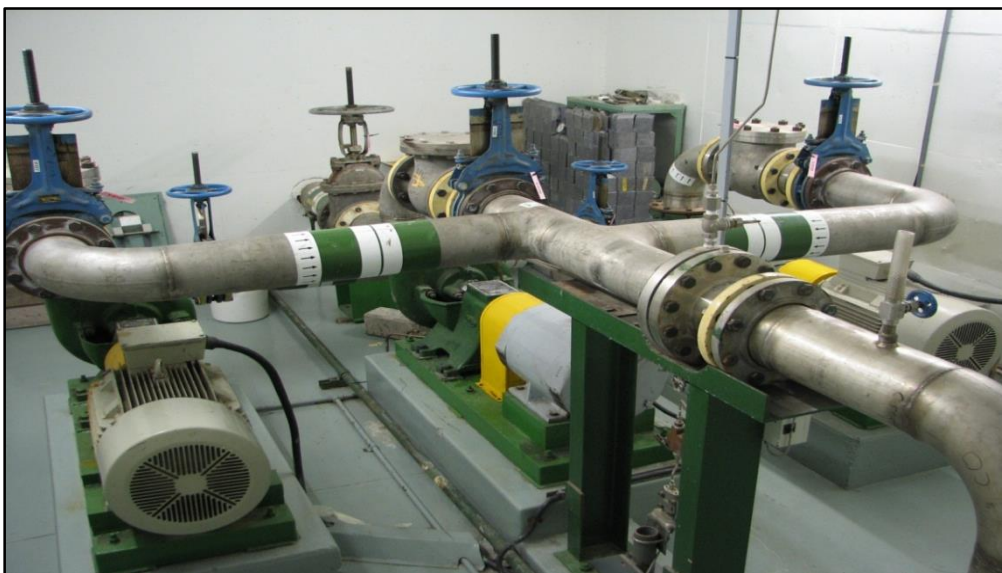
Figure 3 : Pump Room, Showing the Emergency Core Cooling Pumps (the two outer pumps) and the Decay Heat Removal Pump (the middle one)
