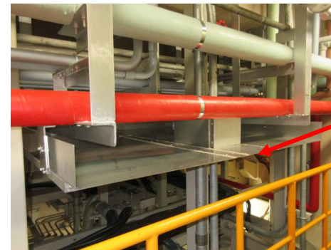
Above power supply panel
